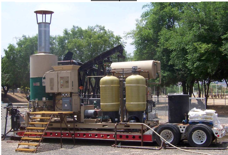
20 mmbtu Steam Generator to be commissioned
