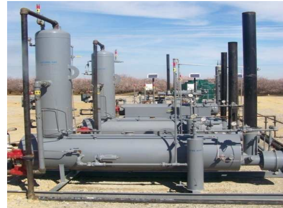
SELH 3 well gas production facility
