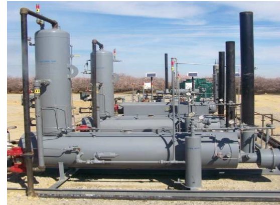
SELH 3 well gas production facility
